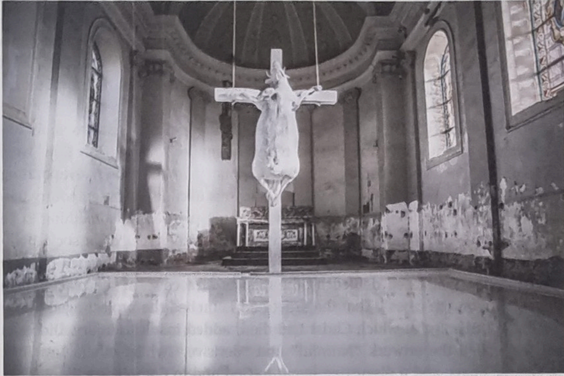
Fig. 1: Tom Herck's installation 'Holy Cow' in the former parish church of Kuttekoven in the Belgian province of Limburg, 2017. Despite its abysmal state, the building's function as a previous place of worship is evident. Photo by Erik Jamar. Kindly reproduced with permission of the artist.
